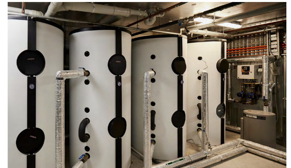
Heat pump systems. Image by Kim Landy.
