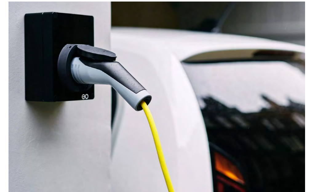
Electric passenger vehicle charging. Image from www.evse.com.au .
