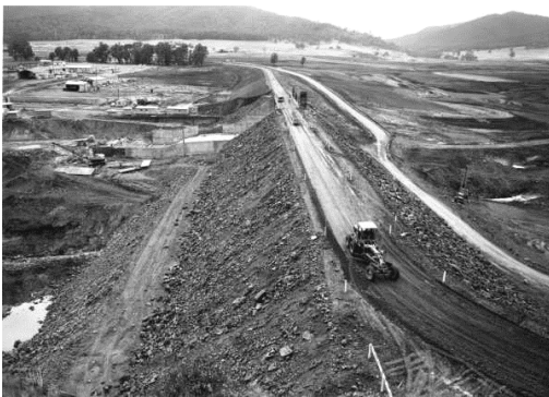
Building the dam wall for Lake Buffalo, 1965 (photo © State Library of Victoria).
